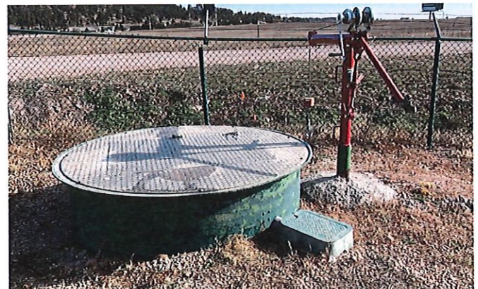
Southwest Lift Station
