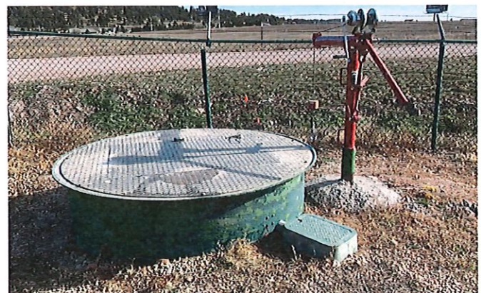
Southwest Lift Station
