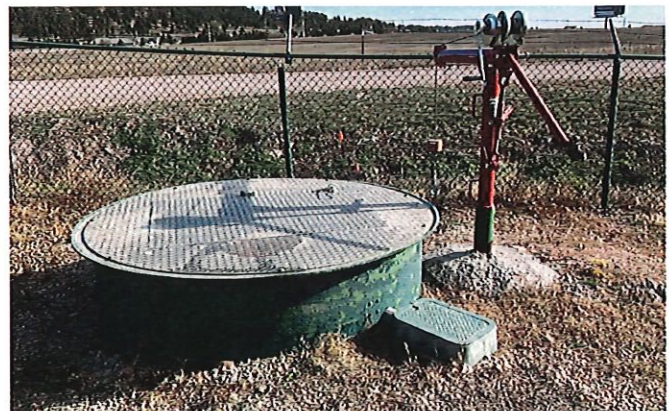
Southwest Lift Station
